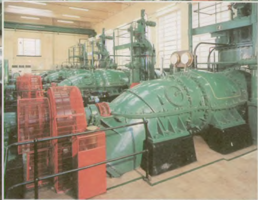
The pumping station interior
