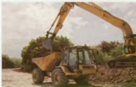
Engineering clay being transferred to a rear tip dumper fitted with low ground pressure tyres to prevent ruts being formed on the bank top.
