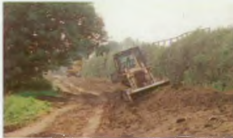
A drott being used to shape and compact the engineering clay of the flood bank
