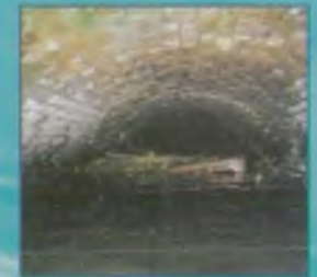
Potential blockage of culvert
