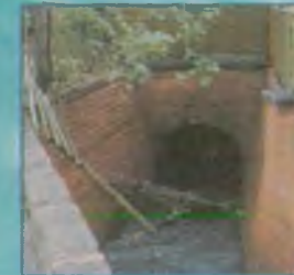
Poor access to channel
