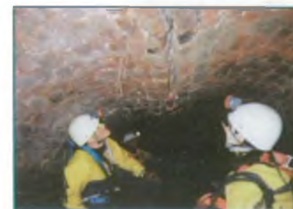
Typical condition of a poor section of culvert
