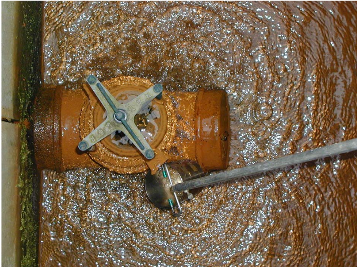
Figure 3.17 Sampling of an outlet level control structure used in the Whitworth No 1 wetland
