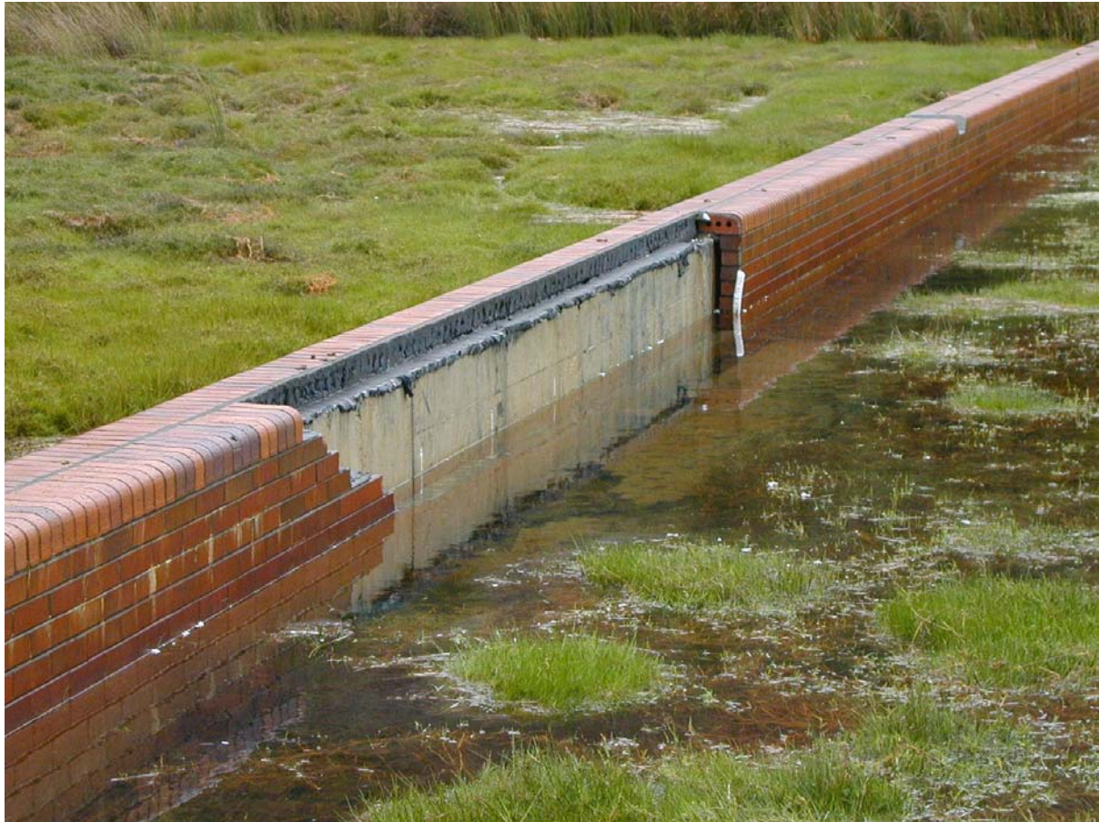
Figure 3.18 Physical damage of the brickwork at Garth Tonmawr
