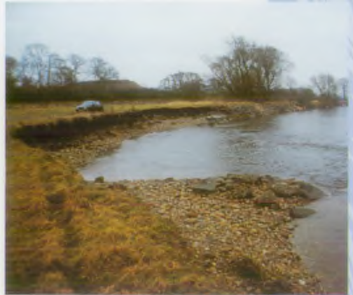
4. A groyne was built into the channel to deflect the current away from the bank. Unfortunately the opposite effect occurred and the erosion was exacerbated.
