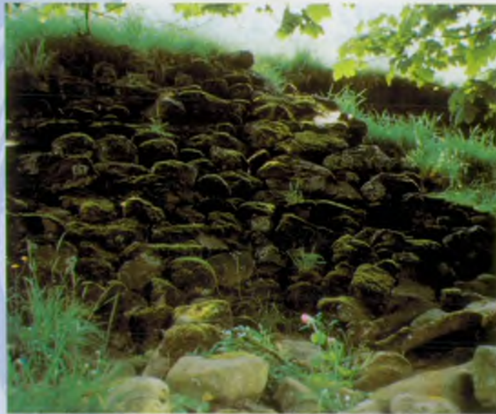
7. Examples of pitching can be seen in the Yorkshire Dales today, still in a good condition after 150 years or more.
