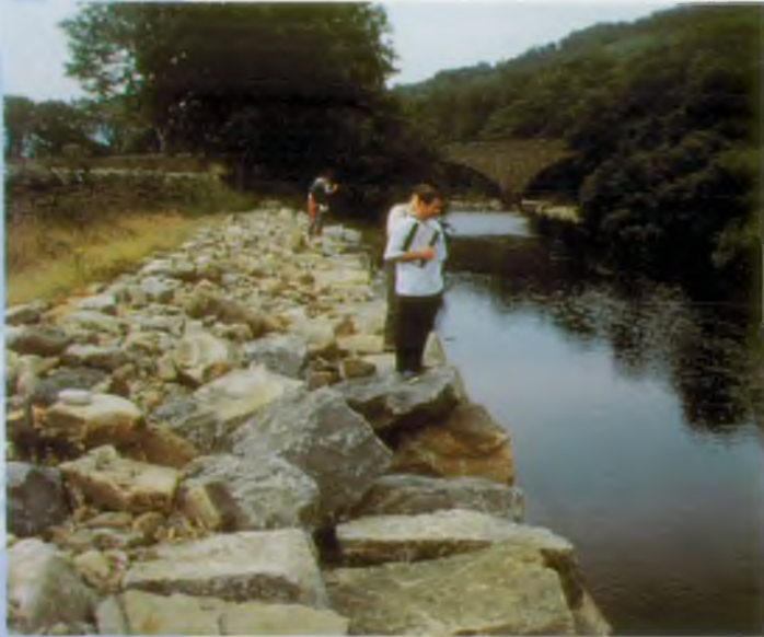
6. This 'hard engineered' scheme was costly and is being undercut after only two years.
