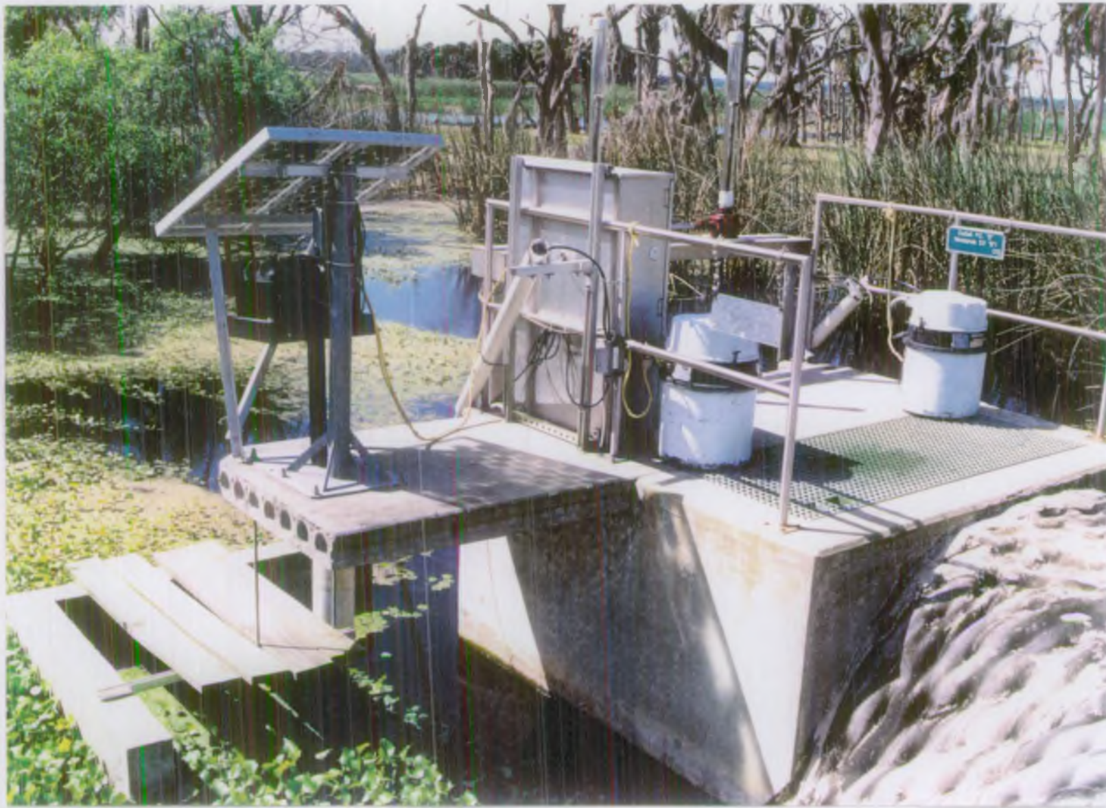
Outfall control and instrumentation at City of Orlando Wetlands Reclamation Project.
