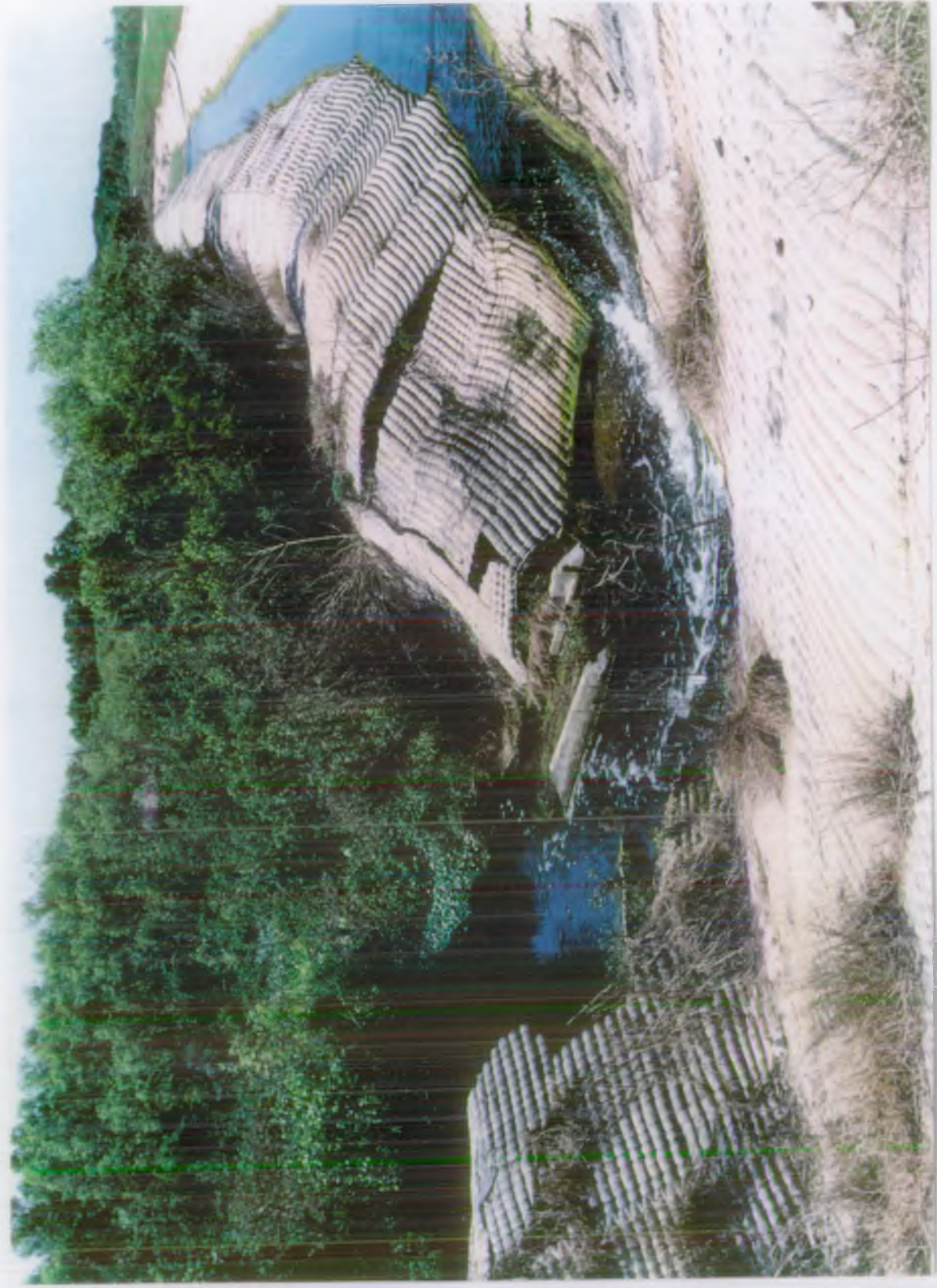
City of Lakeland Wetlands Project. Collapse due to construction over fine tailings.
