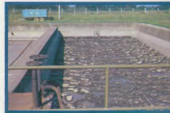
Modernisation of sewers and sewage works will help to secure clean rivers.
