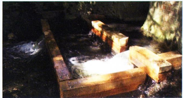
Figure 5: The timber baulks bolted to the road culvert apron create a series of pools and increase water depth through the culvert.
