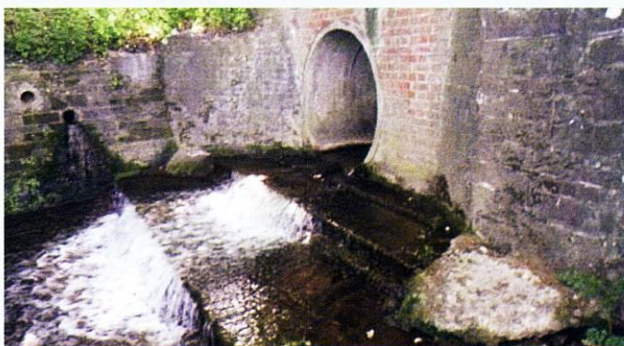
Figure 4: The impassable culvert on the Sussex Ouse tributary, before the easement went in.
