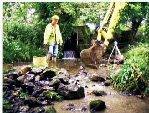
Figure 6: Local block stones being lowered into the channel ready to form the core of the pre-barrage on the Adur tributary.
