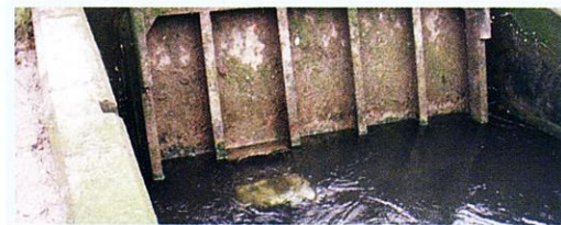
Figure 2: the impenetrable-looking tidal gate at the mouth of the Stiffkey; the silver structure in the middle of the picture is a cat-flap fish pass
