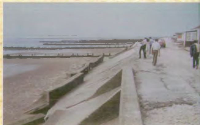
Damage caused by storm tide in 1978
