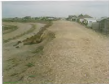
Snettisham – Poor state of the shingle ridge
