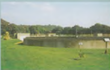
Launceston sewage treatment works
