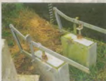
Double locked valves on a circular slurry tank
