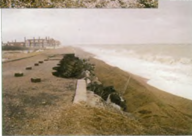
Sandwich Bay storm damage – winter 1996
