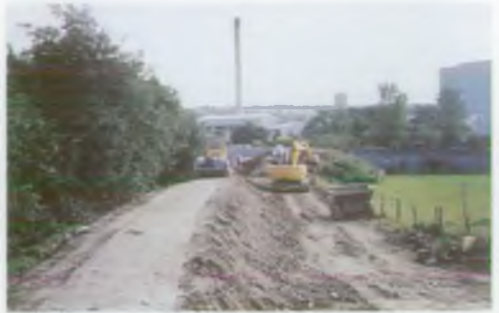
Work in progress - River Gronw floodbank on playing fields north of the A40.
