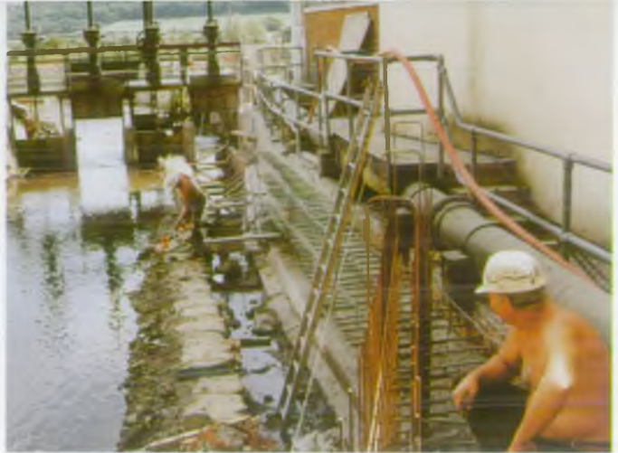
Work in progress showing difficult working conditions, restricted access and complex services arrangements within Creamery site.
