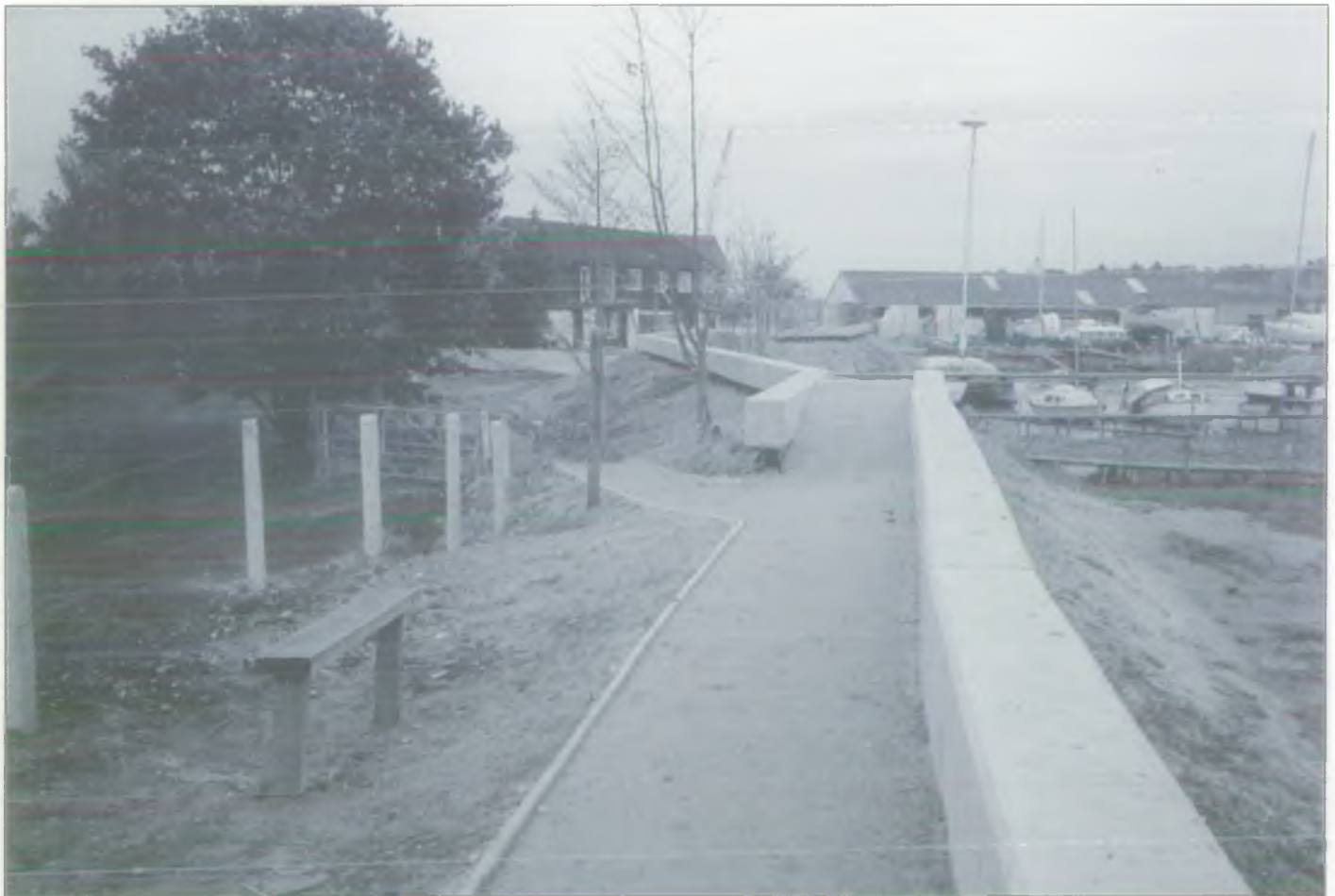
Above: New concrete capped steel sheet pile defence, Tide Mill Yacht Harbour.
