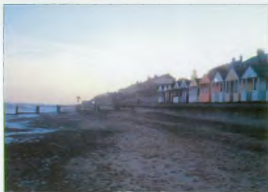
Groynes in poor condition and not providing intended function.
