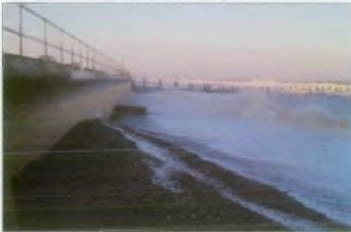
Ineffective groynes contribute to low beach levels that threaten seawall stability and lower amenity value.
