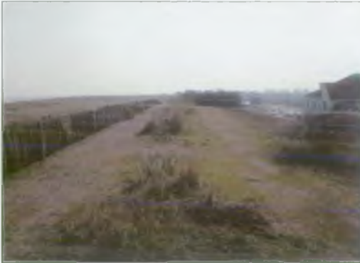
The back face of the Denes - seepage has occurred in this location that could cause instability of the back face.
