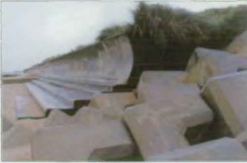
Erosion of cliffs beyond the seawall is raising the risk of failure by outflanking.
