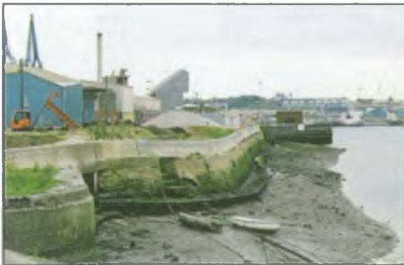
Failed defence at Velocity Control Structure
