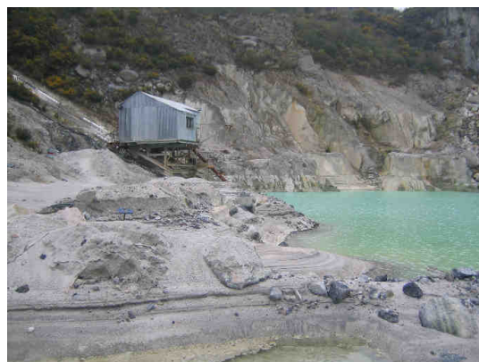
Photo A9.40 Sump pump mounted on rails
