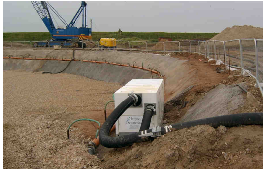
Photo A9.49 Wellpoints with suction pump
