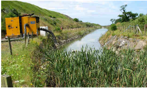
Photo A9.17 Settlement ponds in treatment area on north side of site
