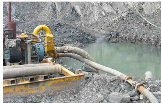
Photo A9.20 Minor sump with pump; pipeline leading to vapour masts and attenuation ponds
