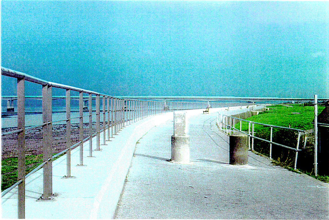
Plate 11 : Walkway on New Wall Severn Beach, showing access control structure to prevent access for vehicles
