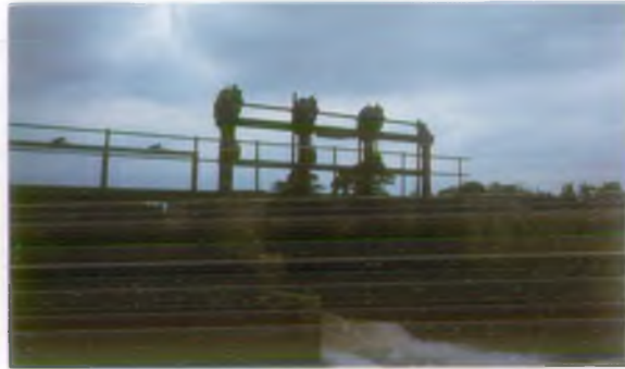
Control structures: an integral part of service provision
