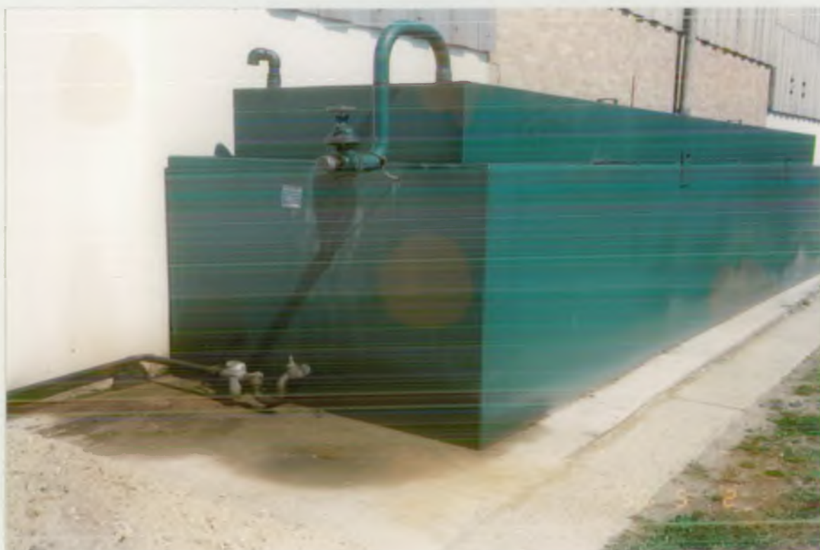
EXAMPLE OF FILLING POINT OUTSIDE BUNDED OIL TANK
