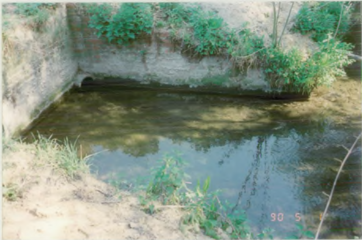
MAIN SURFACE WATER OUTFALL, MILL LANE IND. ESTATE, ALTON (1.5.90) (AFTER POLLUTION PREVENTION SURVEY)
