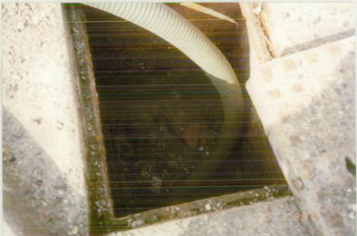
CONTAMINATION IN SURFACE WATER MANHOLE
