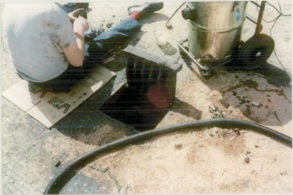
CONTAMINATED SURFACE WATER GULLEY BEING CLEANED
