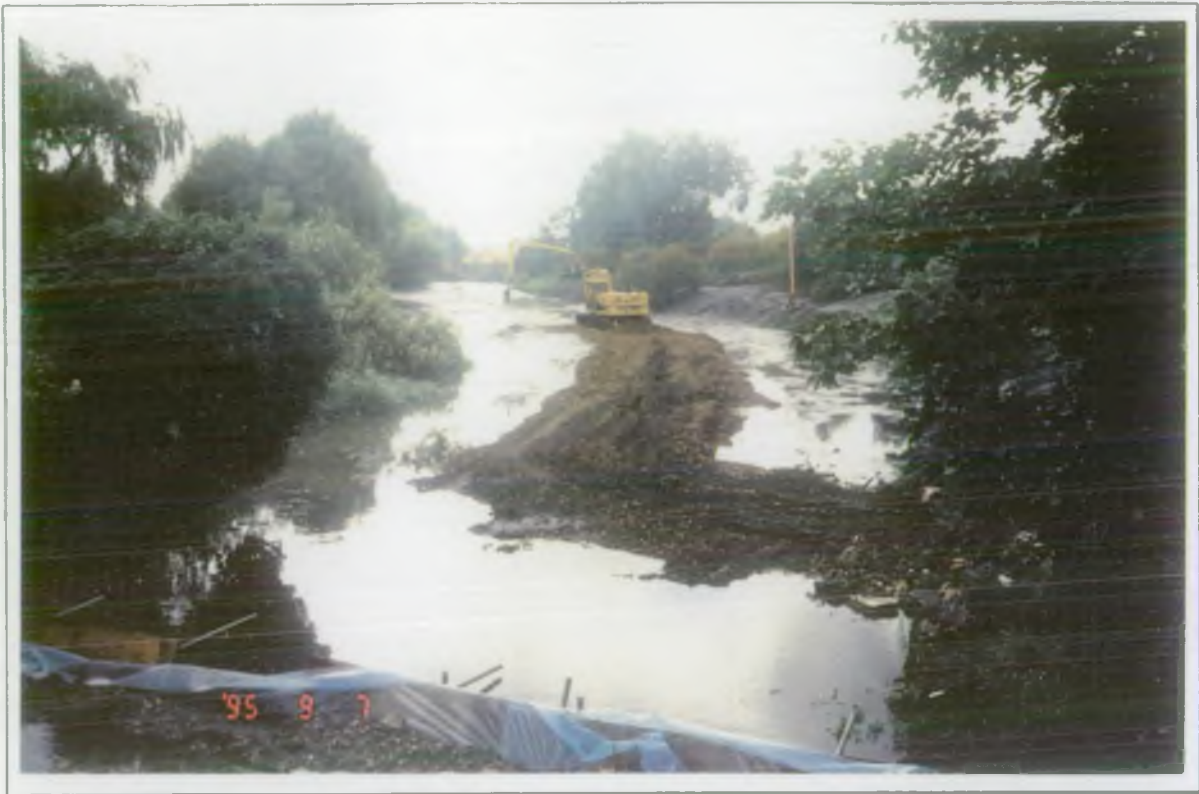
Gravel rejects causeway being built along route of new low flow channel, 7 September 1995
